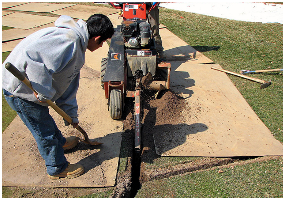
Improving the infrastructure by installing sand-channel drains improves drainage in old topsoil-based greens. Improved drainage is good for the grass and definitely aids in firmness.
