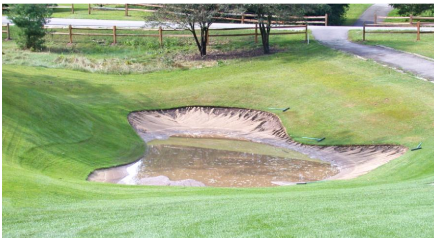
Converting this sand bunker into a grassy hollow makes sense, but simply replacing sand with grass will not address the inherent drainage problem in this site. Installing drainage in grassy hollows is no less important than ensuring adequate drainage in bunkers.
