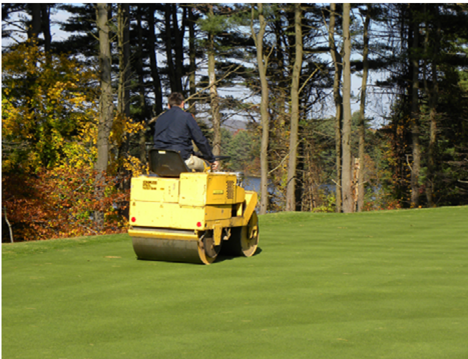
Rolling is an important process in establishing new sod. Rolling with a heavier one-ton roller was initiated after the washed sod was well knitted and stable or about four weeks after installation.
