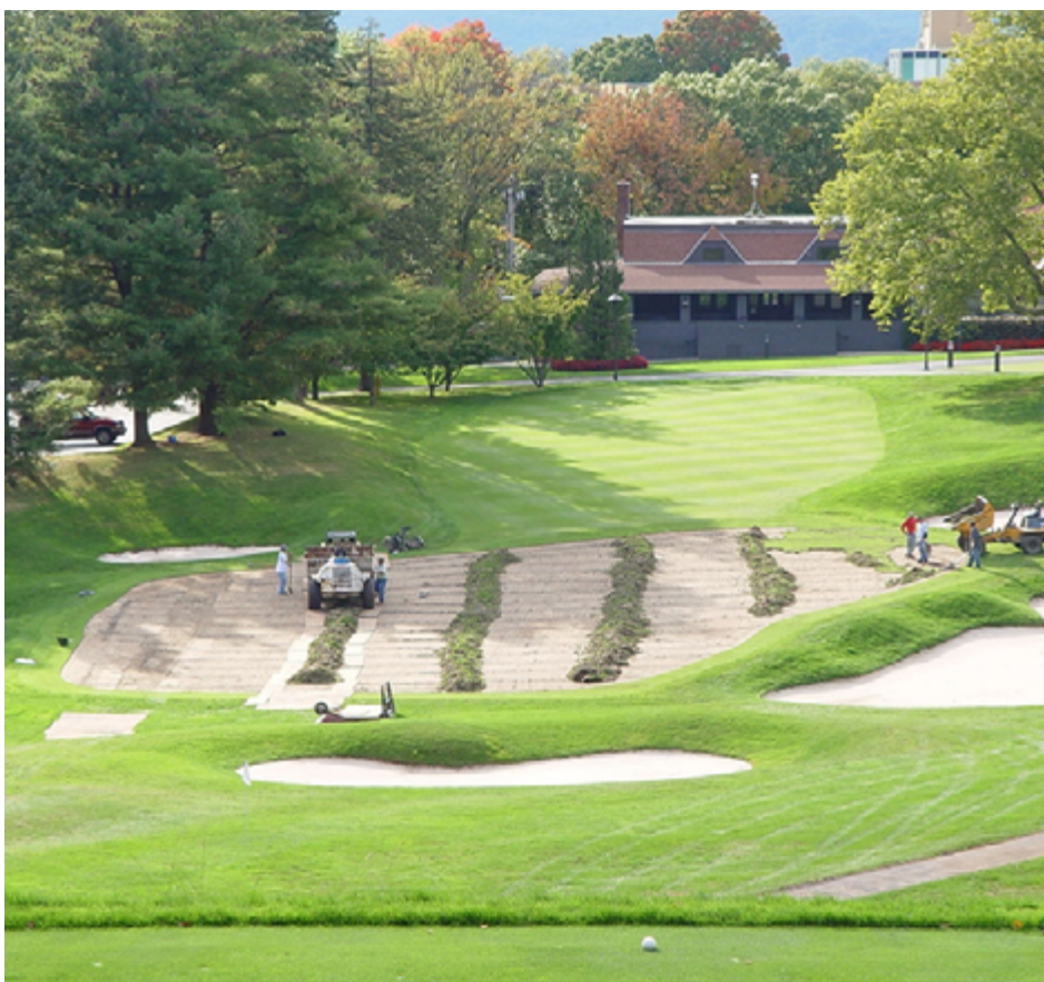
Sod is being removed from a green which can then be cultivated and fumigated prior to installing new sod.
