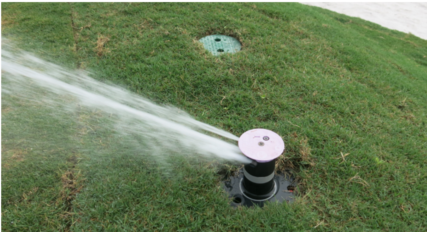
Analyzing irrigation coverage before and after installation can ensure good coverage and help predict the approximate irrigation requirements for each individual green.
