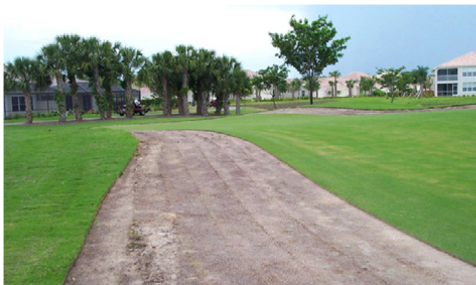
Reducing the elevation of raised collars through aggressive stripping may be necessary to alleviate sand dams around greens.
