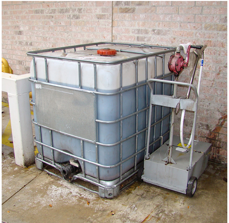
The used cooking oil storage tank is located at the clubhouse. A pallet tank works well in this instance.
