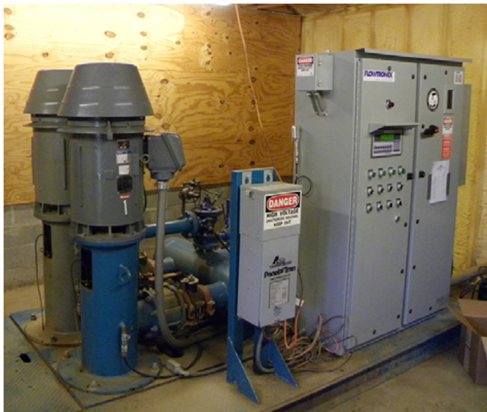
The pump station provides the power to push water through irrigation pipes and eventually through the irrigation sprinklers in each area of the golf course.
