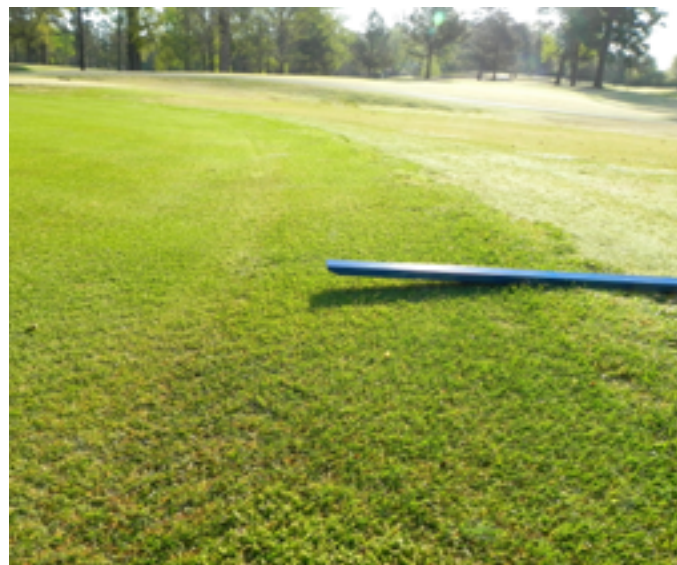
Collar dams are often overlooked as a significant impediment to surface drainage. Regrading affected areas to promote positive surface drainage can eliminate a problem that affects playability and turfgrass quality.
