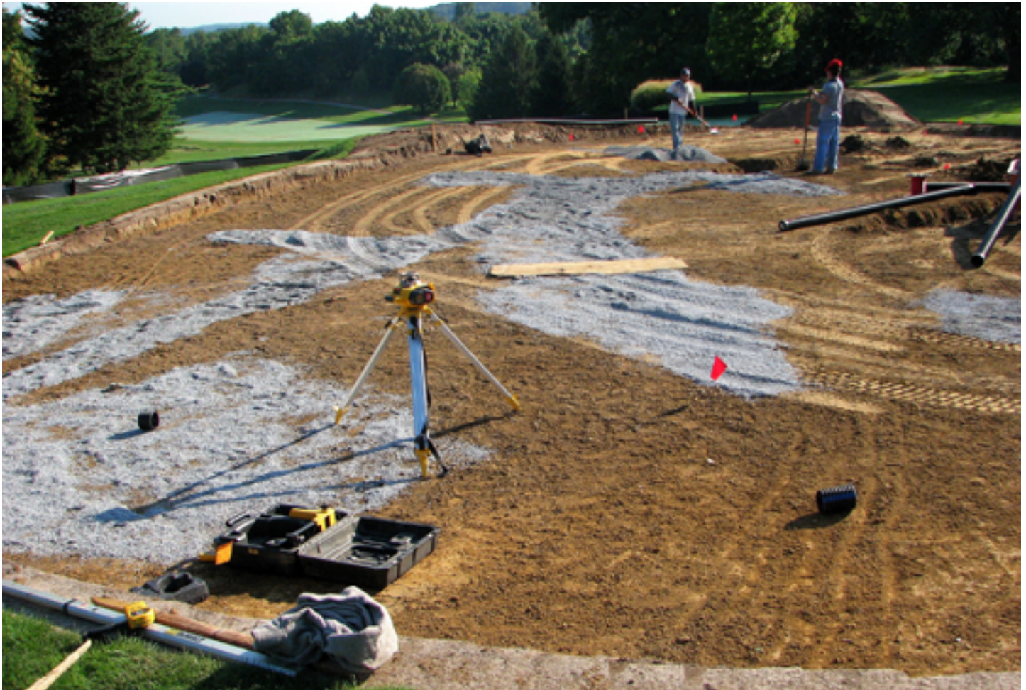
Total renovation of putting greens is an expensive proposition, but it offers the opportunity to address factors that limit putting green performance from the ground up and can provide dramatic long-term improvement.
