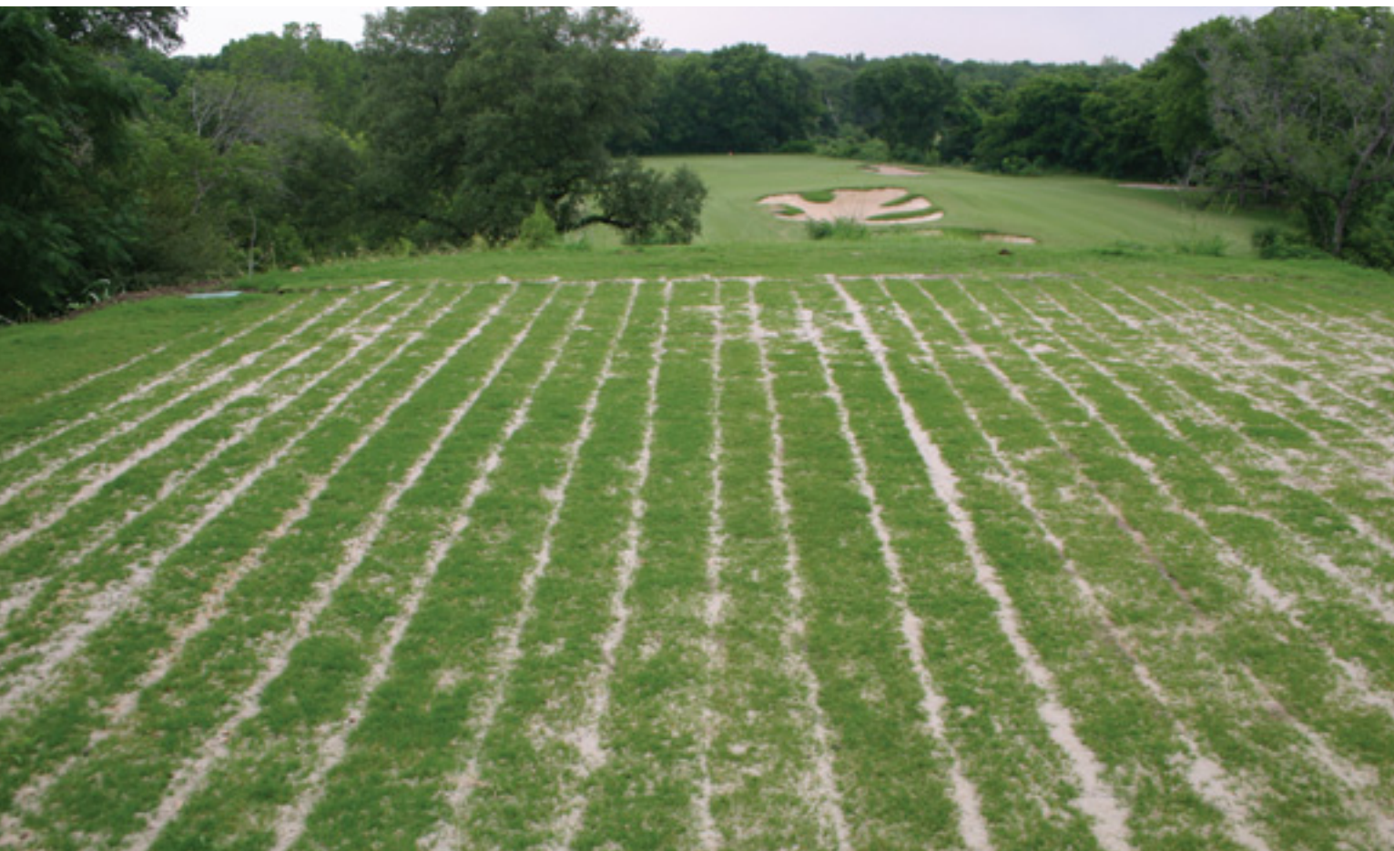
Converting an overhead irrigation system to a subsurface drip system is a project that can be accomplished in-house with the right tools.
