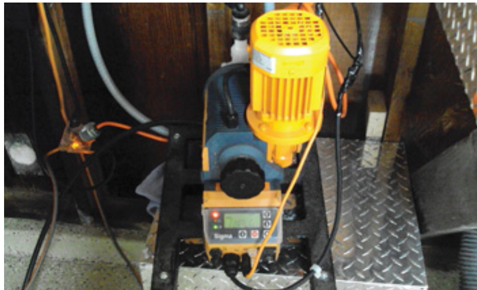
This pump is used to deploy N-pHuric acid into the irrigation water when the flow from the pump station exceeds 300gpm.
