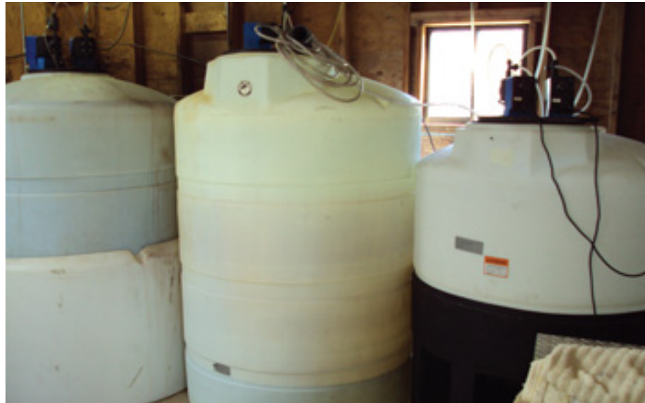
Acid, fertilizers, and wetting agents commonly stored in the pump house may offer better water quality, improved infiltration, and enhanced turf nutrition when injected into the irrigation system.
