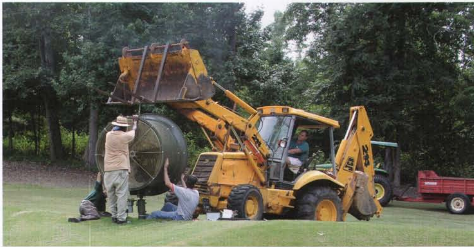
A backhoe or front-end loader easily lifts the fan for assembly to the fan pole. A fork attachment on the loader is a plus to help lift and maneuver the fan. Remember, some type of device also will be needed to transport the fans on and off the golf course for off-season storage.
