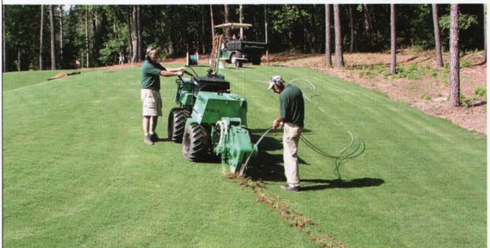
Wire materials and installation are the most expensive costs for a fan project. Installing the wire to the proper depth and according to local electrical codes is essential to supply consistent power to fans.
