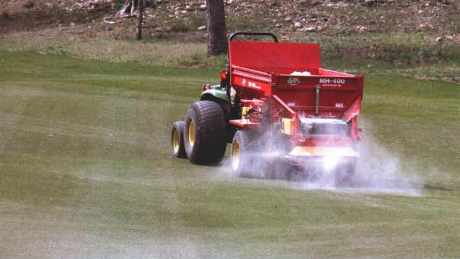
When significant amounts of sodium are present in the soil, typically it is necessary to apply a calcium-based soil amendment, such as gypsum, at routine intervals. Custom application on a frequency of two times per year can cost approximately $30,000.
