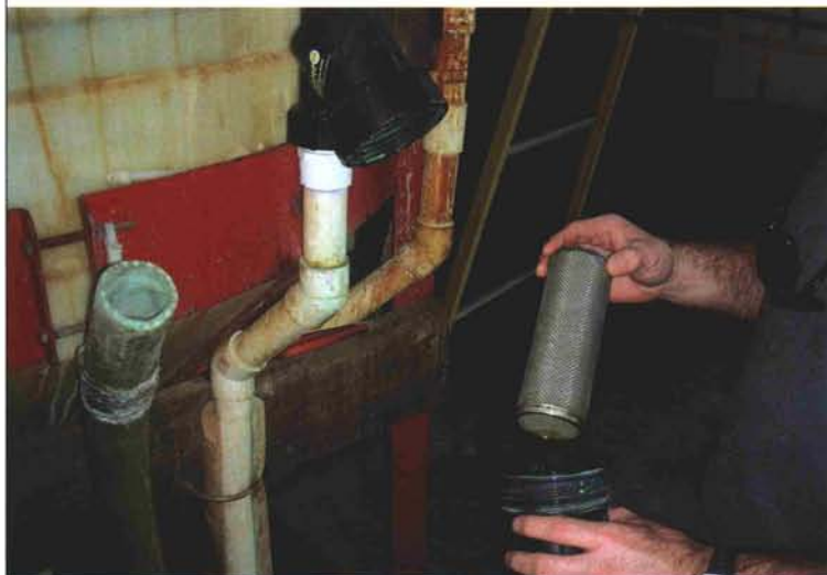
In-line filters are installed in both the tank's fill and discharge lines. Plugged nozzles in the sprayer are a thing of the past.
