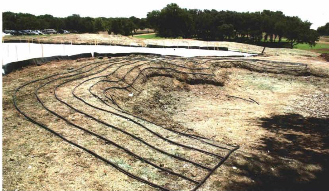
A subsurface drip irrigation system was installed in the grass face of the bunker adjacent to the experimental green. This allows the turf on the face to be irrigated without overwatering the adjacent areas.
