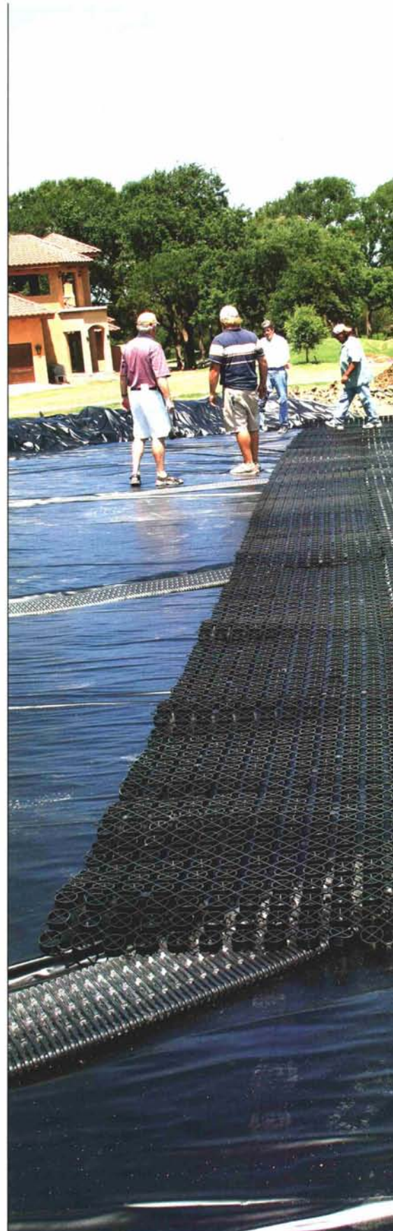
Each half of the experimental green is drained with material drainage blanket normally used in USGA greens.
