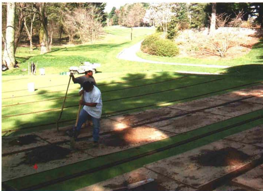
Installation of internal drainage in older, soil-based greens greatly improves their chances for survival in general, but especially under poor weather conditions with wet patterns and high temperatures.
