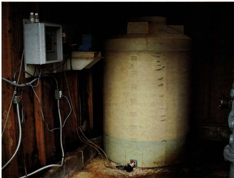
The direct injection of sulfuric acid into the irrigation mainline from a nearby storage tank is another method to introduce acidifying amendments. The hazard of handling concentrated acid must be considered along with the need to provide adequate space at the pump station for the storage tank and access by delivery trucks.
