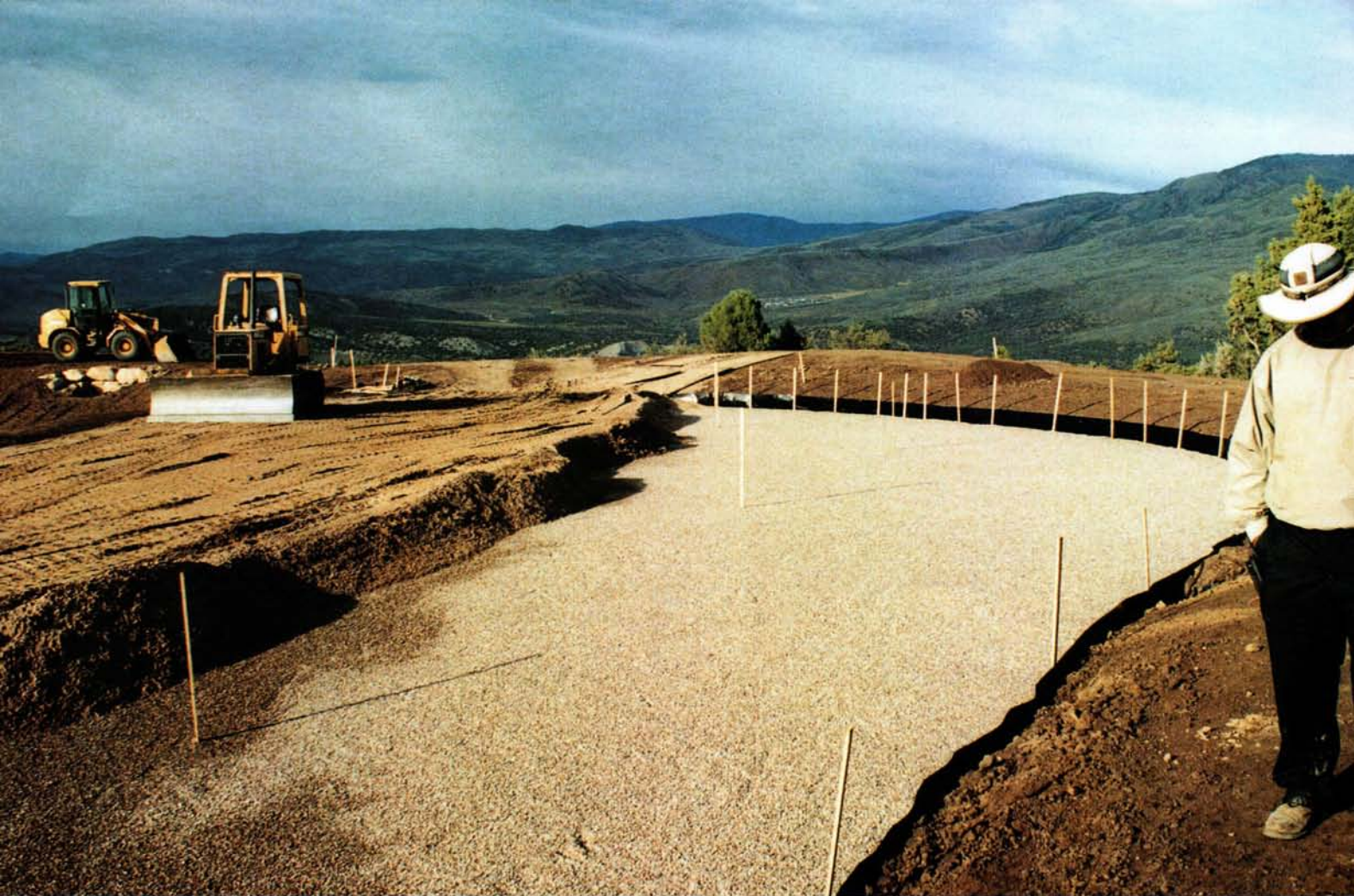
Building putting greens is a costly endeavor, involving specified materials and several construction steps. Soil amendment selection can significantly affect the bottom line.
