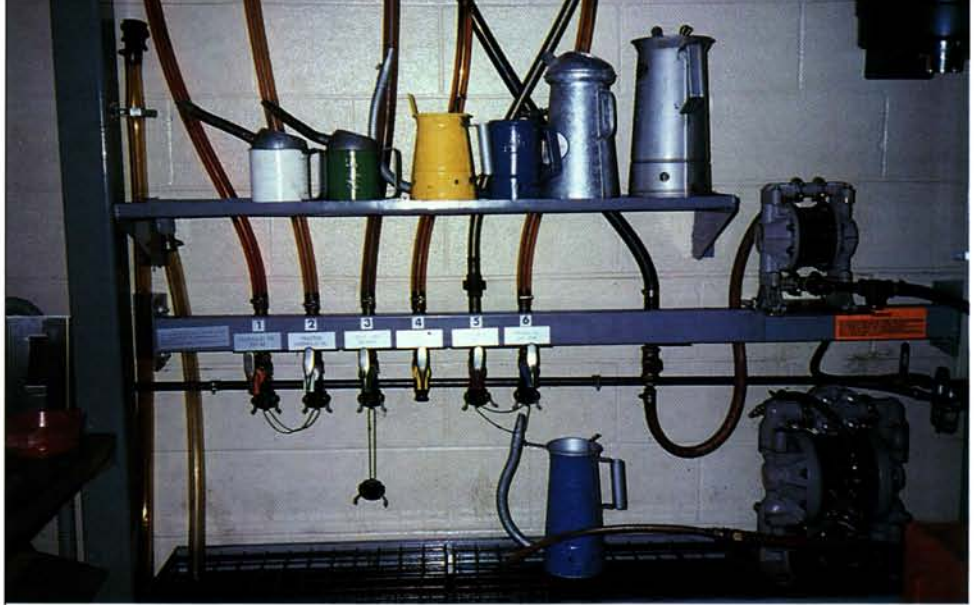
Bulk oil dispensing can be clean and efficient. Oil is dispensed from six steel drums. A drip trough catches any spillage.
