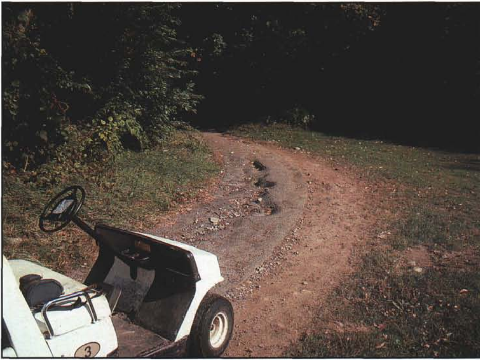
A golf course owner or operator has a duty to exercise reasonable care for the safety and protection of others. Daily inspections of the golf course help to identify potential hazards. This inspection is a critical component of a risk management plan.
