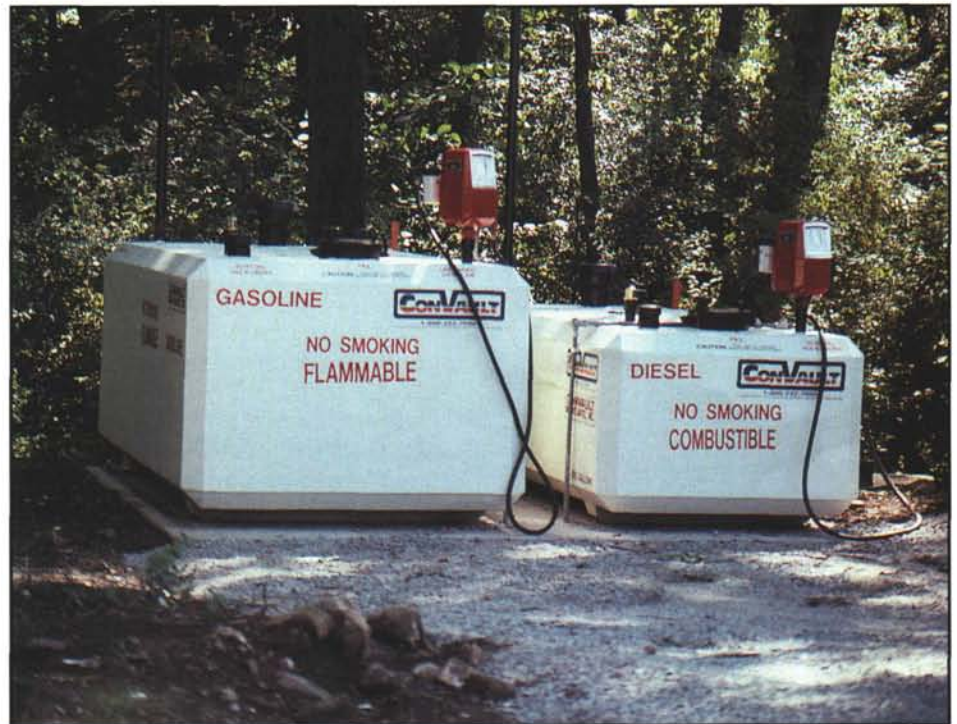
Properly designed fuel storage tanks demonstrate the facility's commitment to safe and environmentally sound operations. These tanks are in the initial stages of installation.
