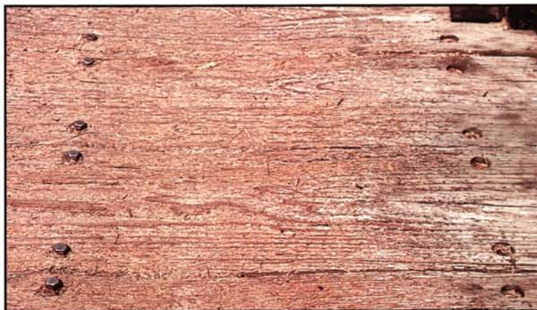
Metal spikes can cause significant damage to non-turf areas. The counter-sunk bolts on this bridge have been exposed as metal spikes have worn away the wood on the trafficked portion of the bridge.
