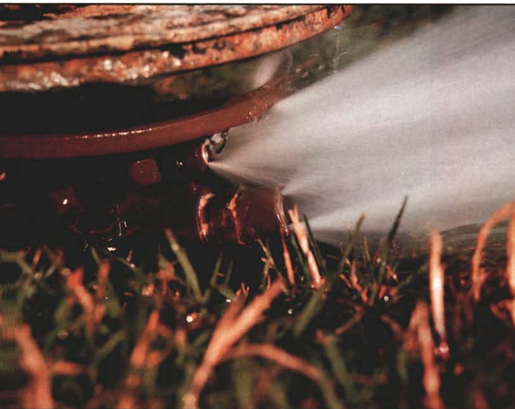
The patented insert's notches strip a small amount of water from the main stream, placing it close to the sprinkler head, without affecting the distance water is thrown.
