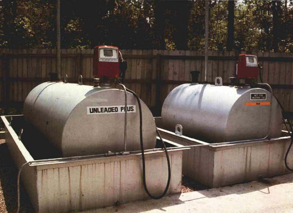
It's better to replace old tanks before they cause problems. Fuel tank storage can be improved by the use of safer and cleaner alternative tanks that are available on the market.
