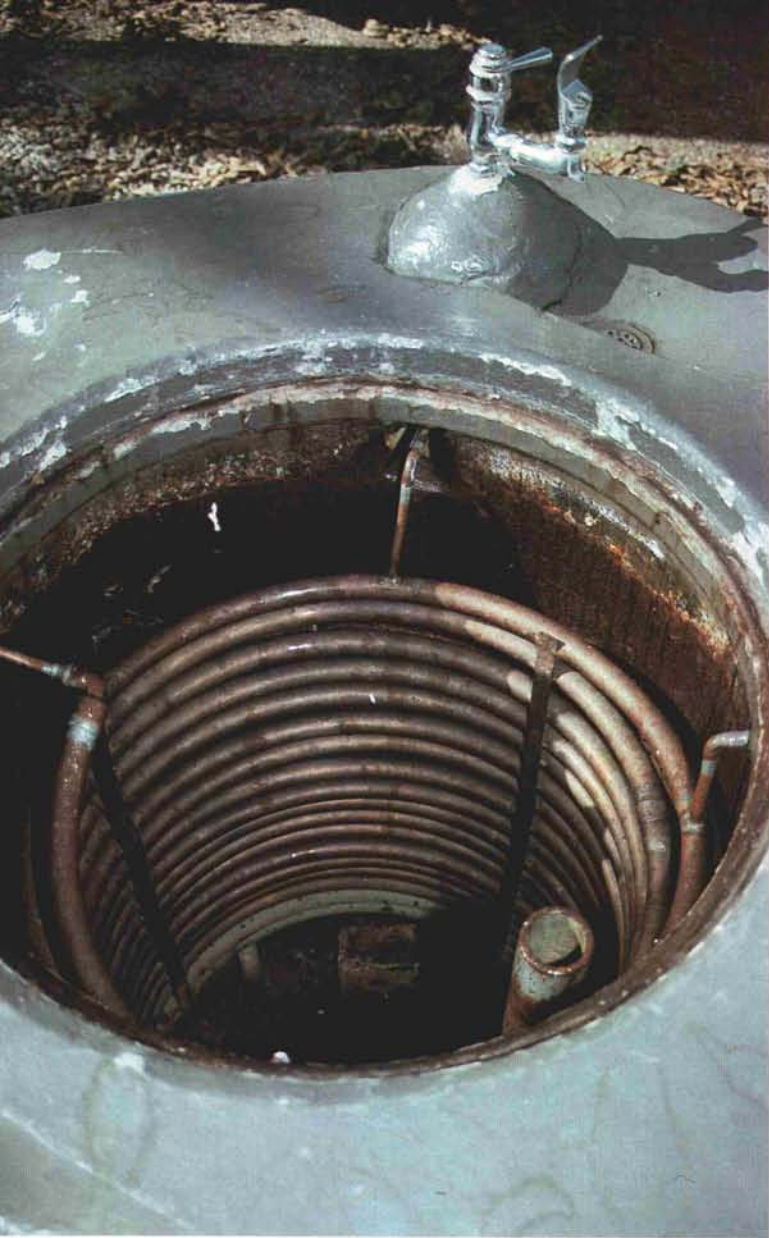
A continuous coil of 1" copper tubing brings water from the supply to the fountains.
