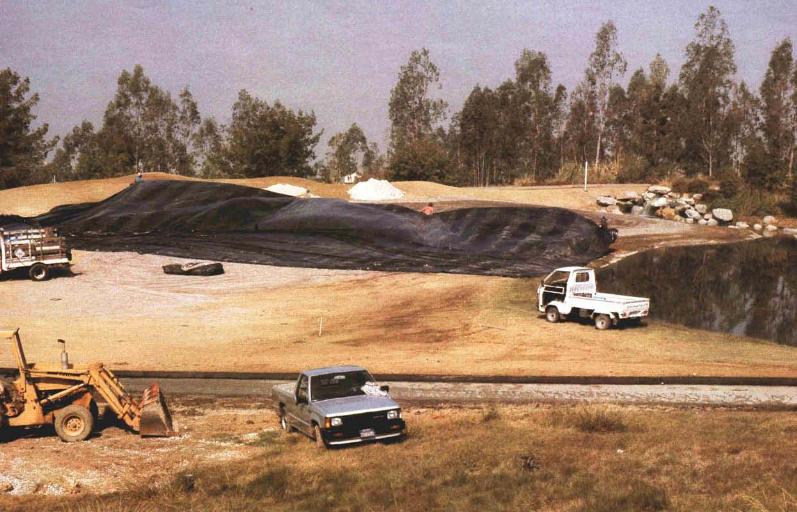
At the Industry Hills Golf Courses, a chlorinated polyethylene liner was installed beneath a methane-affected green to prevent gas migration into the root zone.
