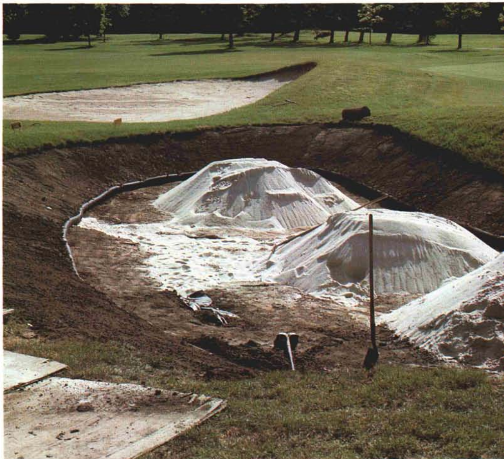
During the Acacia Country Club bunker renovation, drainage pipe was used to delineate the renovated bunker edge.
