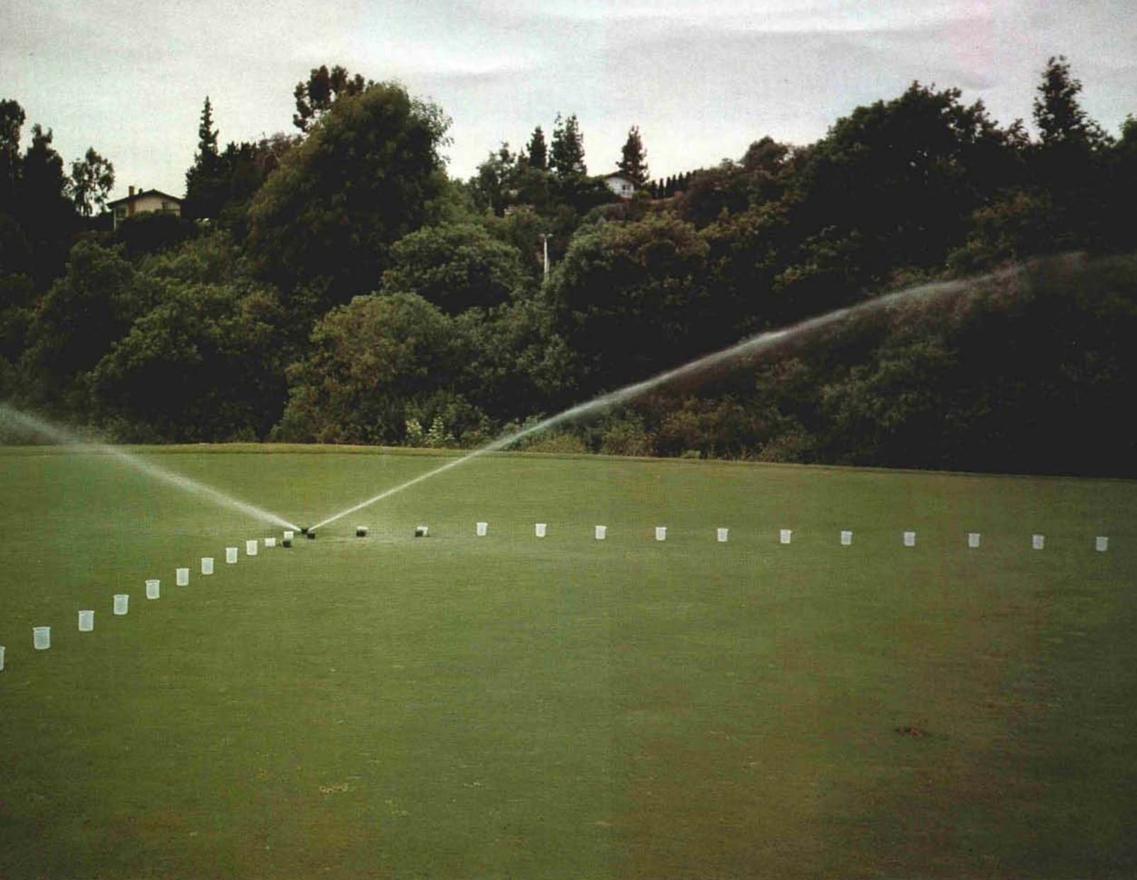
When installing a new irrigation system, selection of a particular sprinkler head model should be based solely on performance. Evaluation requires measuring the amount of water distributed at regular intervals away from the sprinkler head and then analyzing the data with special computer software.
