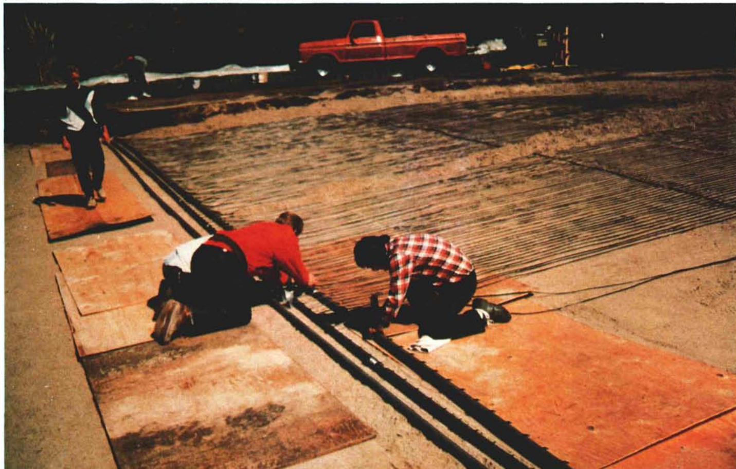
Stay alive at 55°. A constant soil temperature will be maintained year round on the 5th green with the installation of the sub-surface heating systems.
