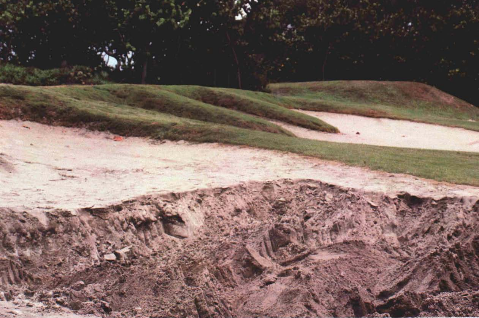
Over three-and-a-half feet of sand was removed from No. 13 green front bunker and the grass fingers reshaped to the original height.
