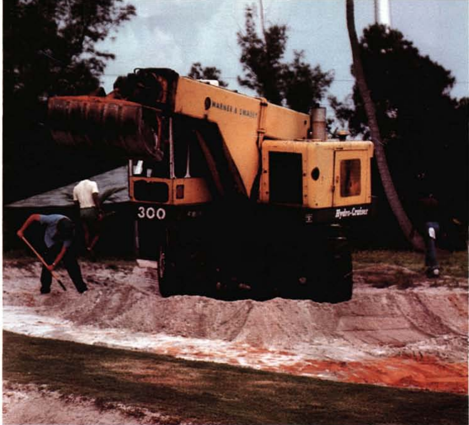
A critical factor in the bunker sand removal was an experienced Gradeall operator.
