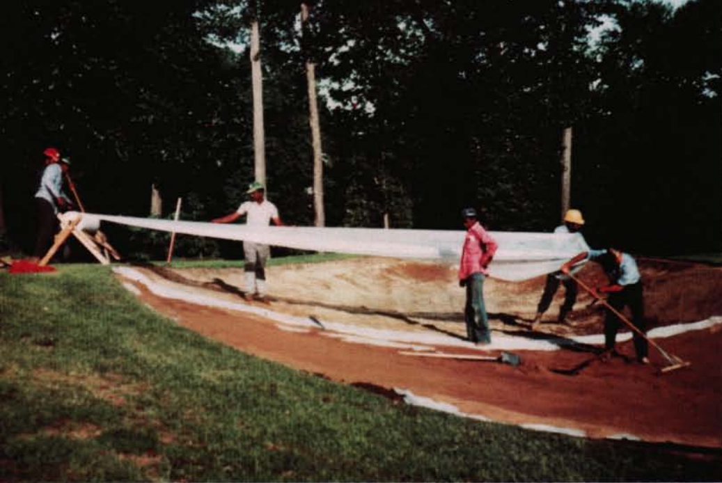
Measuring and placing the nylon cloth in the bunker base. Its purpose is to keep the new sand from being contaminated with rocks as a result of winter freezing and thawing of the underlying soil.
