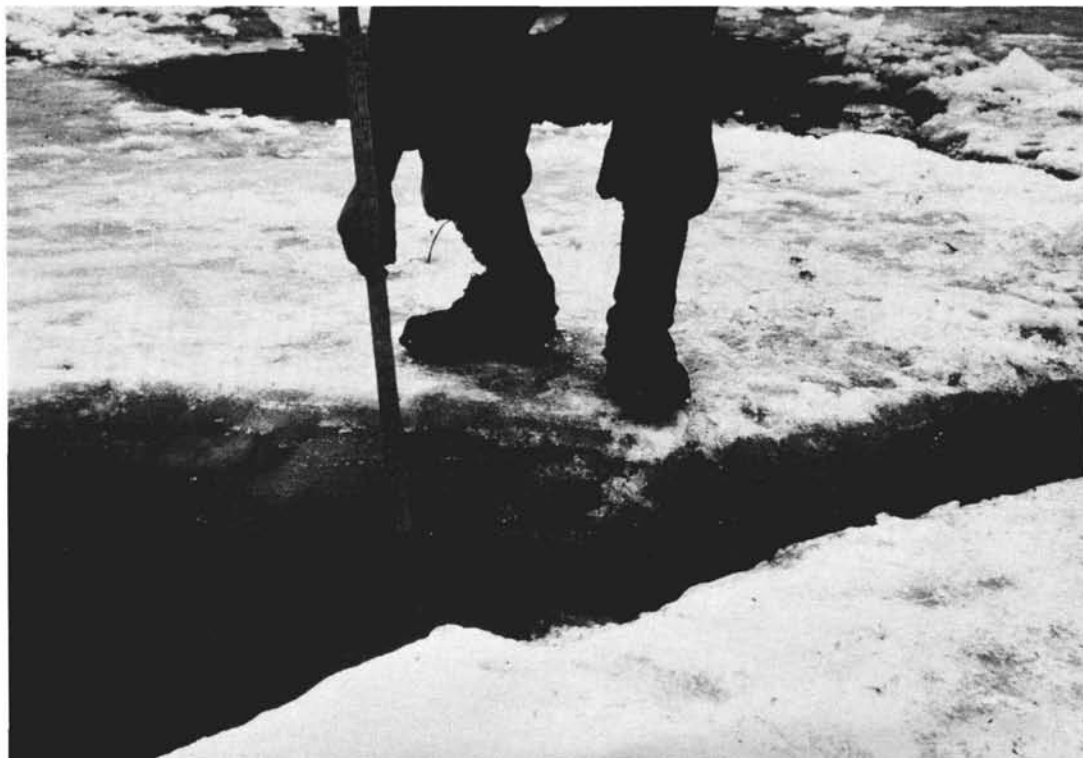
A water main leak in freezing temperatures is real winter trouble.
