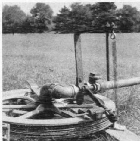
Fig. 2—When control valve closes irrigation stops.
