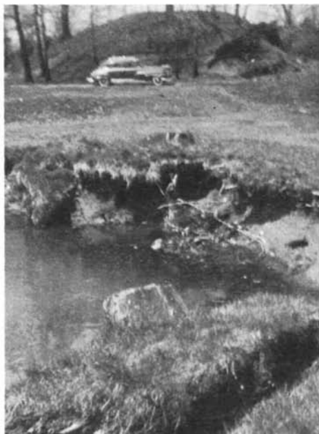
A close-up of erosion of the banks of the brook at the fifth hole, third nine, Montclair Golf Club, Montclair, N. J.
