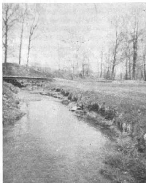
Members are often unaware of erosion and deterioration because it is out of sight or below the surface of the ground.
