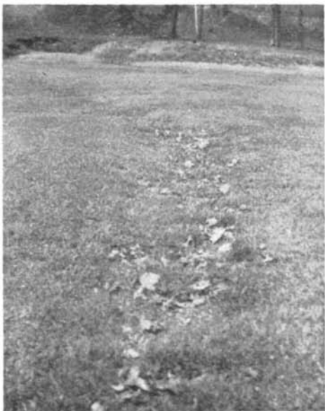
A sunken drain across the middle of a fairway at the Montclair Golf Club caused this depression to appear at the fifth hole, third nine.
