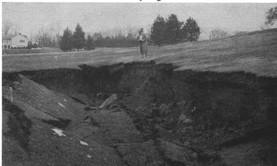
This is what the spring rains did to the eleventh fairway of Woolfert's Roost Country Club, Albany, N. Y. A heavy three-inch rainfall overburdened a storm sewerage line causing it to break. Here, Mr. Jack Gormley, Superintendent, surveys the damage. In some areas of the fairway the soil deposit resulting from the break measured approximately two feet in depth.
