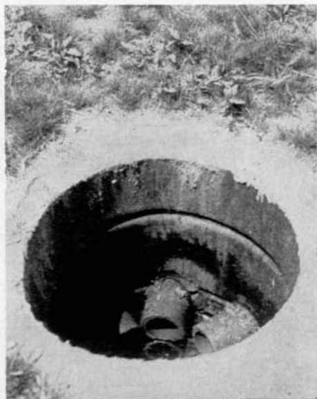
Sherwood A. Moore, superintendent of the Hollywood Golf Club, Deal, N. J., makes good use of discarded herbicide drum in forming catch basins for fairway drainage lines.
