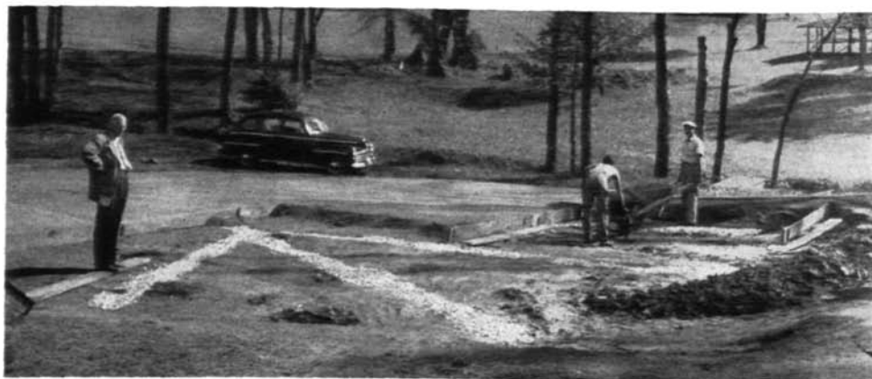
Alex G. McKay, the author, inspects the sub-surface drainage system while workmen haul topsoil. Mr. McKay uses the herringbone drainage pattern and believes whole-heartedly in sub-surface drainage for best results with bentgrass greens in the South.
