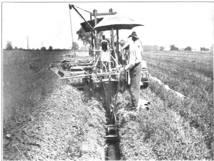
Laying tile with ditching machine. String the tile 6 feet to the right of the ditch line. Use a shield on the machine to keep the ditch bottom free from crumbs. These factors, plus a tile hook, make it possible for one man to keep up with a machine digging 150 rods per day.
