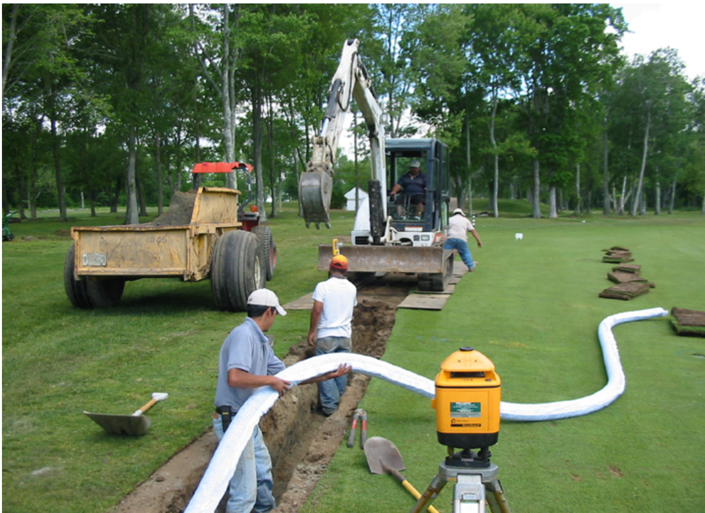
Workers install a 4-inch, wrapped, perforated pipe while a small excavator digs the drainage trench. The trench is checked with a grade laser to ensure a consistent slope. Note that the excavator operates on plywood to avoid damaging the playing surface.
