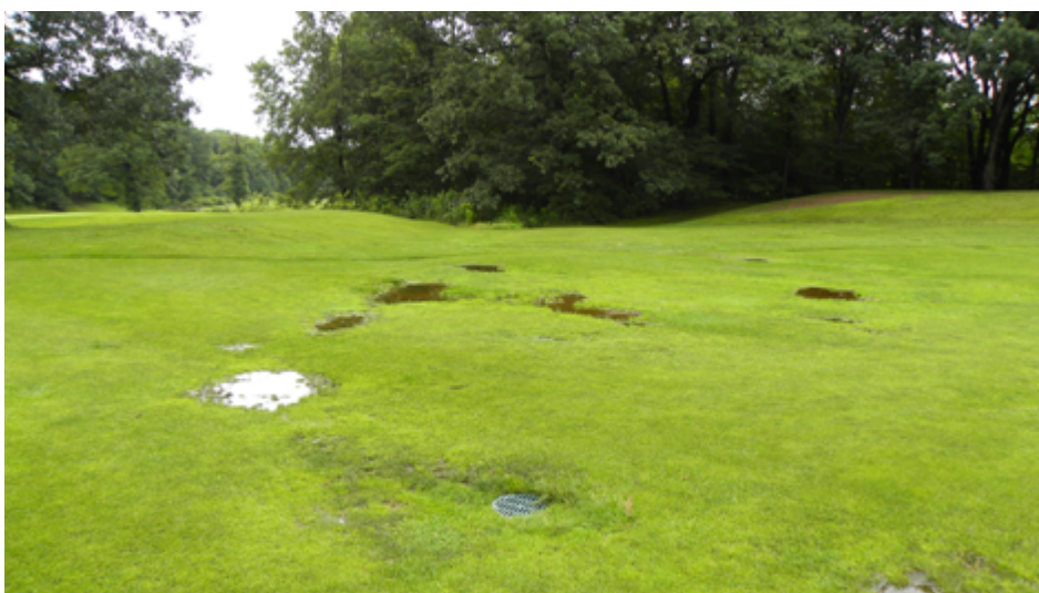
Standing water above a sunken drain line is a good indication that the pipe has failed and needs to be replaced.
