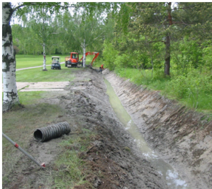
Cleaning open ditches to reestablish water flow maintains a good outlet for subsurface drains and speeds water flow through the property.
