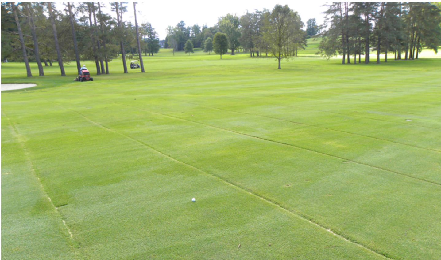
Only a few months after installation, turfgrass has nearly covered the trenches of a slit drainage system. This system follows a grid pattern and utilizes 2-inch, perforated, wrapped pipes in a sand envelope.
