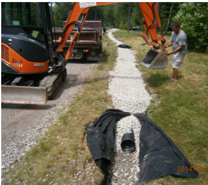
Surrounding a gravel envelope with non-woven geotextile fabric will prevent fine soil particles from migrating into the gravel and perforated pipe.
