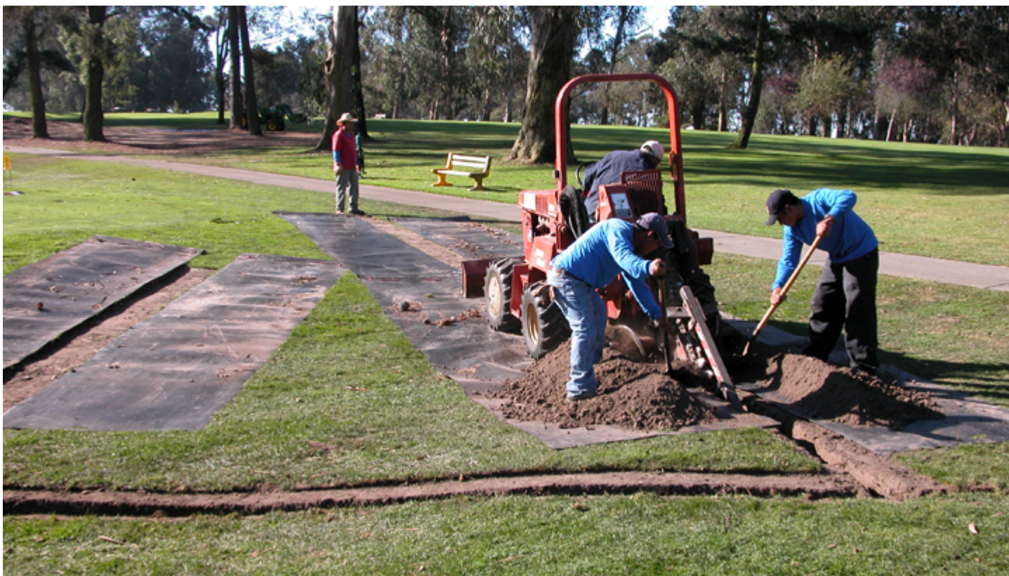
Drainage improvements are an important part of golf course maintenance. Playability and plant health are optimized when there is balance between soil moisture and drainage.
