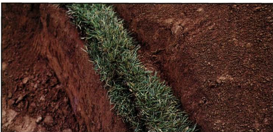
With each layer, soil was added and compacted between the sod and native soil. Tight compaction of the soil behind the sod was imperative to prevent the sod from shifting.
