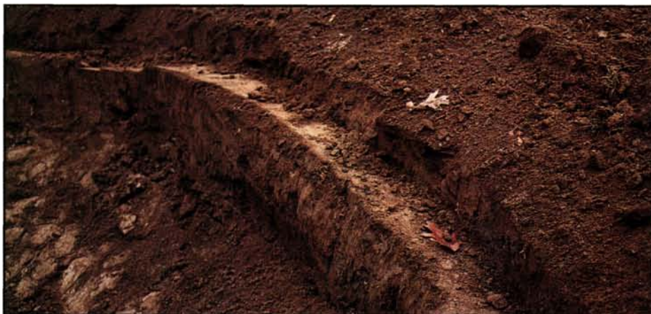
A soil ledge approximately 10 inches in width was created to provide the initial footer to begin stacking sod.
