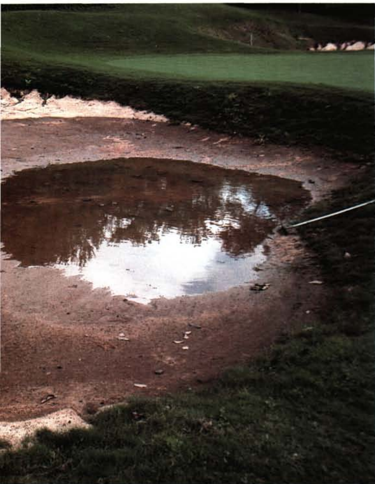
Improving drainage is just one of many reasons why bunker renovation is popular. It's important to be sure the membership understands that the new sand may be "soft" for several months.
