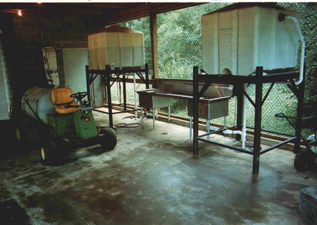
Elevated rinseate storage tanks hold rinseate to be used in the next application.
