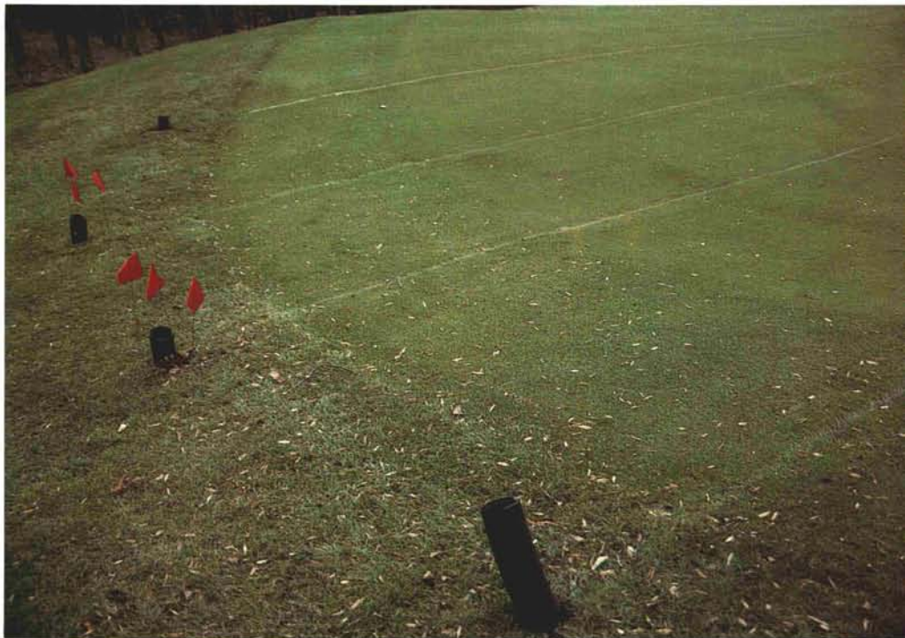
The high ends of the drain lines were brought to the surface, off the green, and eventually were attached to valve boxes for easy access.
