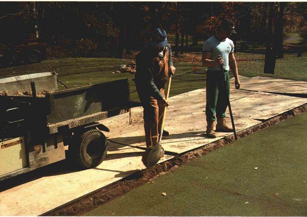
A thin layer of gravel was put in the trench, followed by 3-inch perforated drainage tile and more gravel. Topmix was added and tamped in layers to minimize possible settling problems.
