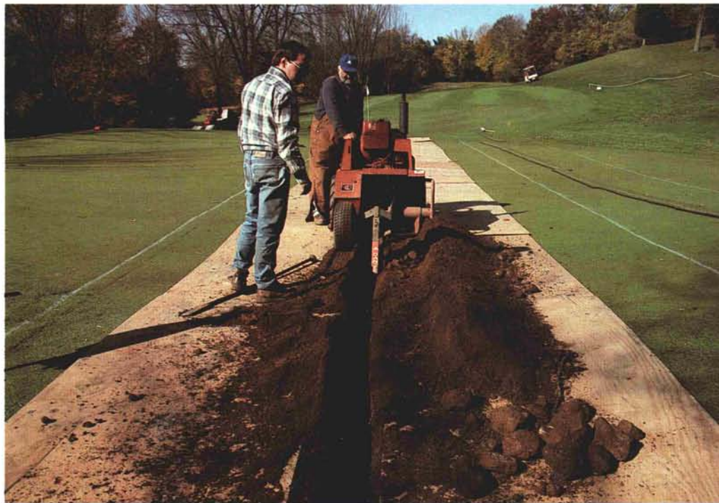
Plywood sheets were laid down along the trench line to protect the turf and make cleanup easy.
