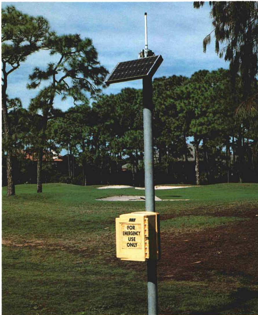
The installation of emergency call box systems on golf courses has been streamlined through the use of wireless communications equipment.
