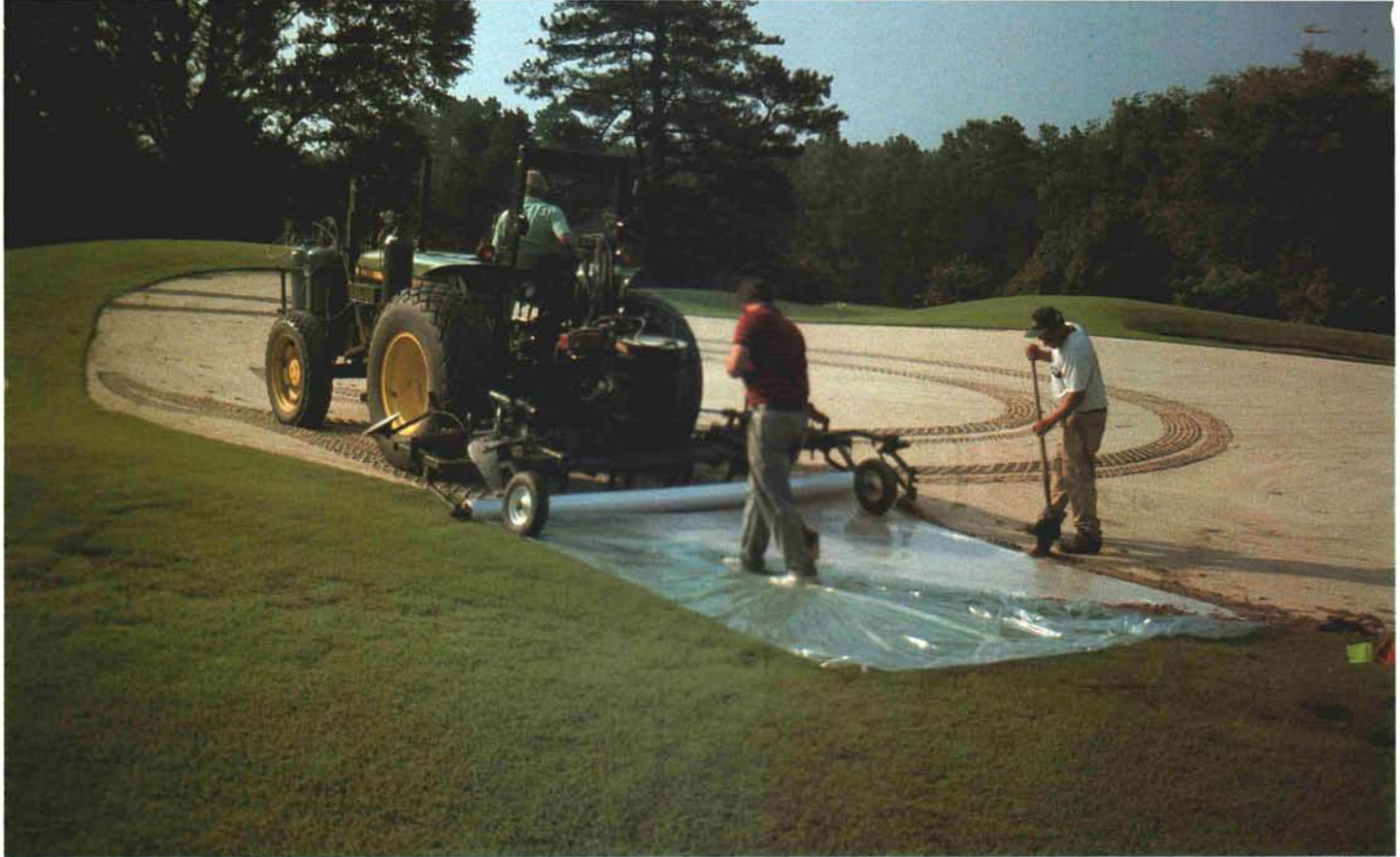
Methyl bromide fumigation was a key step prior to the seed bed preparation. We were convinced this was necessary due to the amount of bermudagrass established during construction on the green cavity wall.
