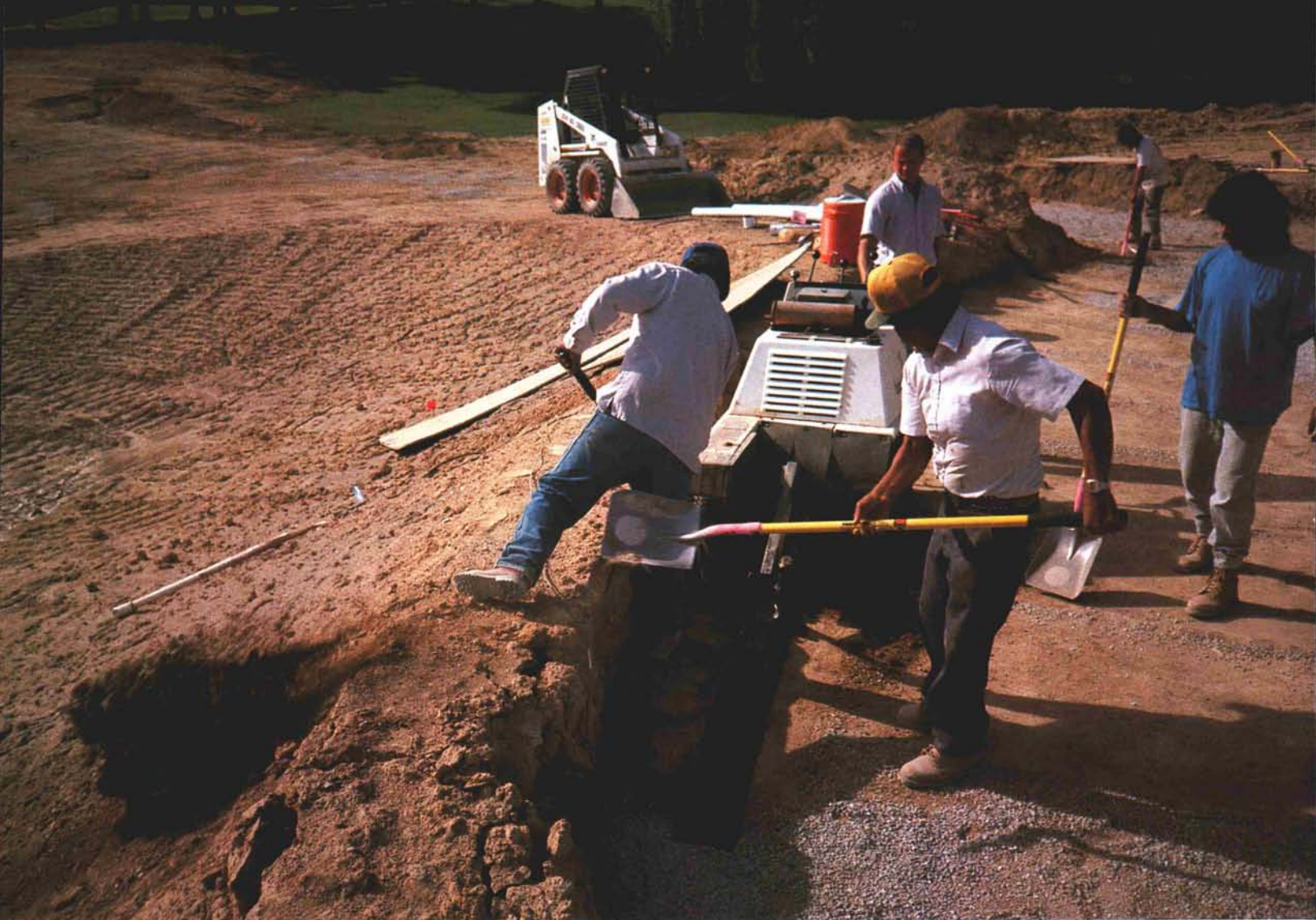
Installation of the "smile" interceptor trench and drain at the low end of a green.
