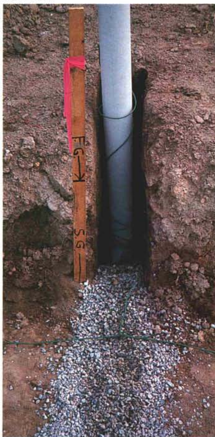
An insulated copper wire, wrapped around the main line, can be used in the future to locate the drainage lines.
