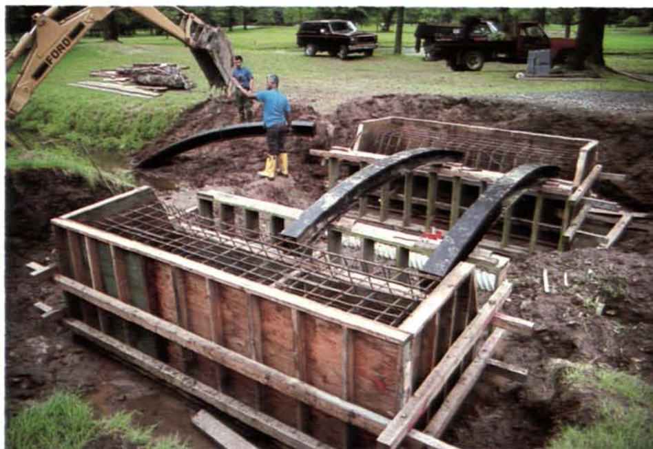
The superintendent's role in managing major course construction projects ensures the best value for the club and its golfers (Upper Montclair C.C., New Jersey).
