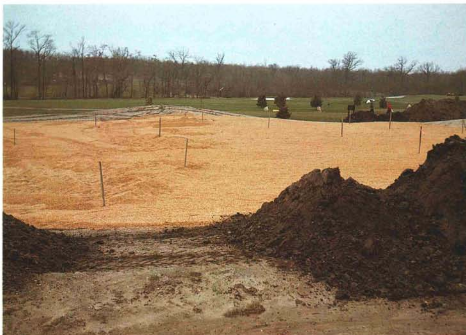
The gravel drainage blanket being laid to the depth indicated on the grade stakes.
