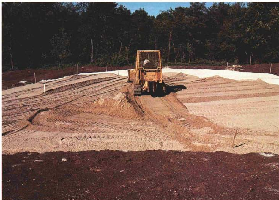
A dozer carefully spreads root zone mix to a depth of 12 inches.
