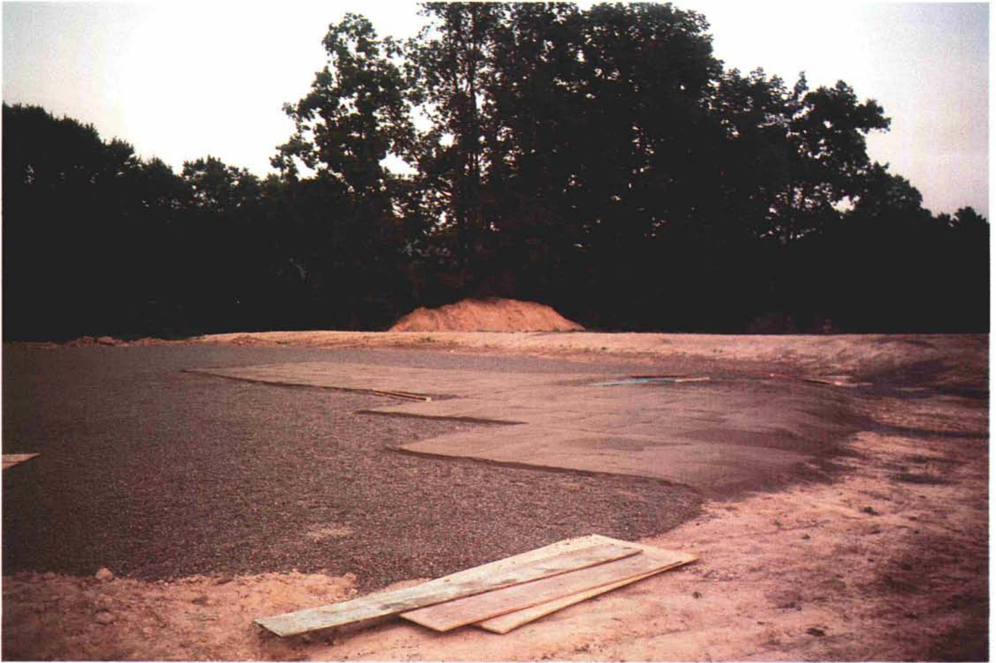
The use of 2" x 4" planks proved most effective for installing a uniform intermediate layer on the new 15th green.
