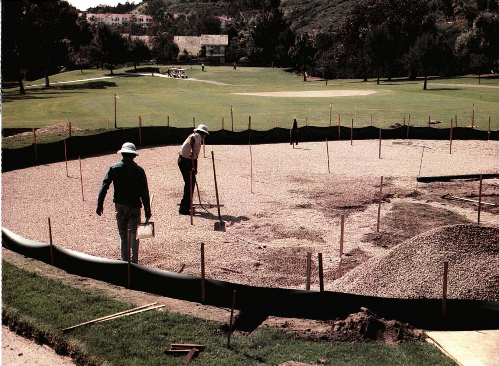
Greens reconstruction can be time-consuming and expensive, but if done properly can provide decades of good turf and cost-effective maintenance.
