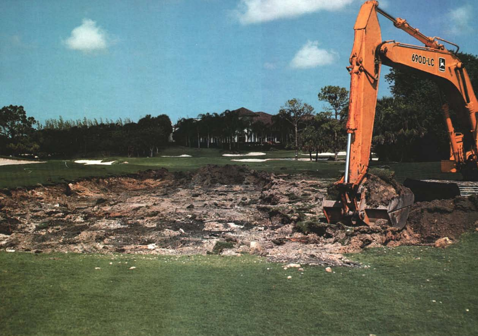
Fairway excavation removed the coral rock and muck soil pockets that previously hindered water percolation through the soil.
